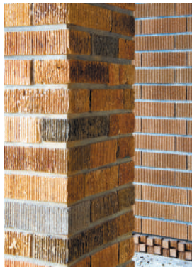
The pillar in the foreground is made from original scratch brick. At the time, brick-makers made the grooves by hand. The pillar in the back is new.
