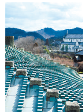
From a distance, the copper roofing resembles Japanese tiles, but when you go out onto the third-floor terrace, you can see how the copper plate has been folded to create the detailed patterns.
