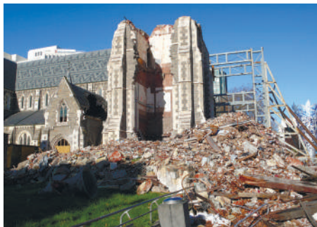
The Christchurch earthquake caused crippling damage to the Christ Church Cathedral.
