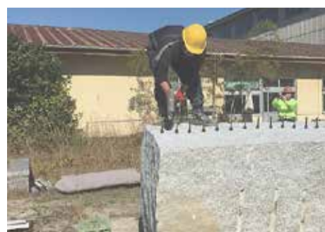
A worker cuts Inada granite, which is used in various buildings in Tokyo. MT. TSUKUBA AREA GEOPARK PROMOTION COUNCIL
