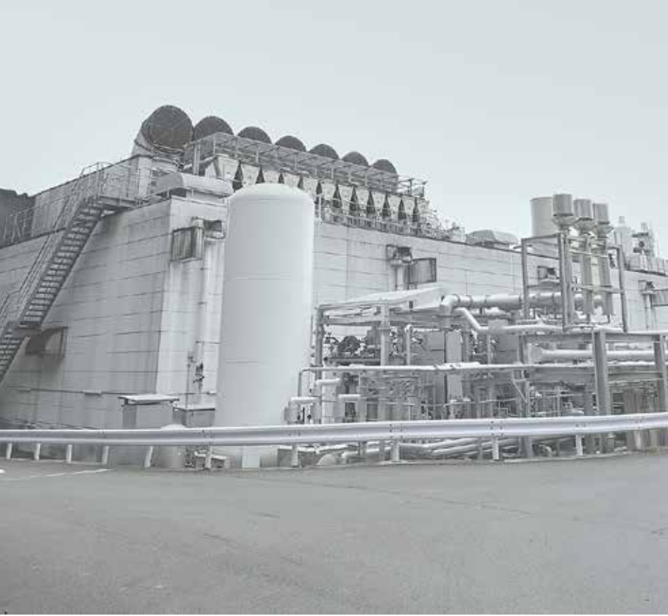
Newly developed high-efficiency, low-pollution experimental hydrogen boilers supplying the Suntory Minami Alps Hakushu Water Plant SUNTORY
